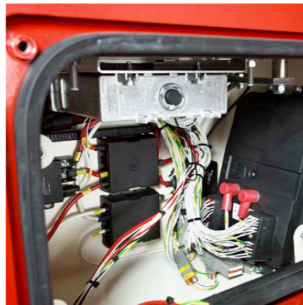
Electric cabinet is easily accessible.
